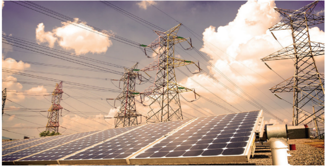
Transmission and distribution, renewables' integration, smart grid applications in the energy sector
